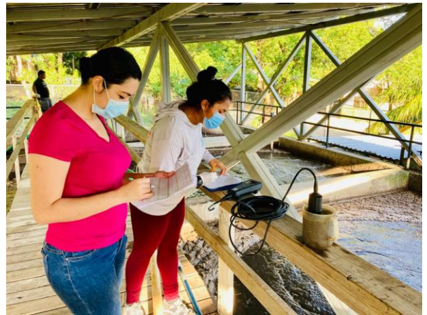
Monitoring the sewage treatment plant in the community of West End, Roatan.
